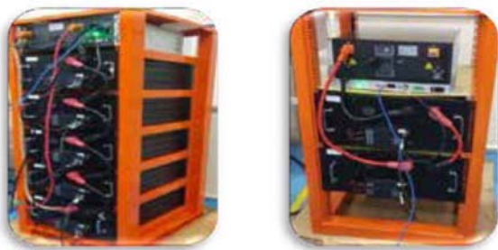
Energy Storage System (ESS)
